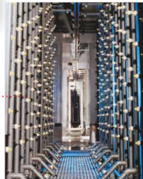
Powder Coat Paint Booth
