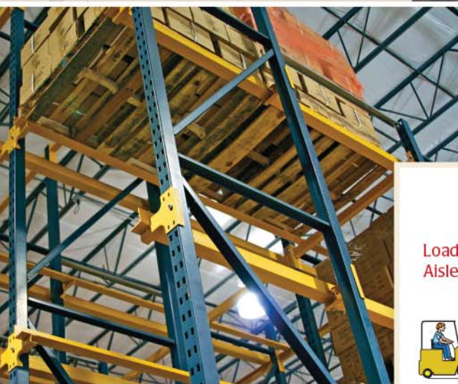
Pallets rest on rails within the bay.
