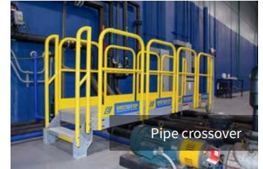
Safe conveyor crossover access
