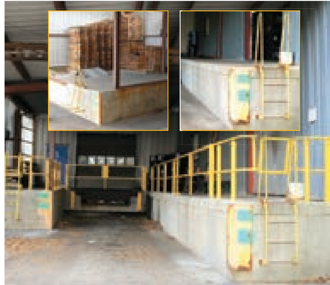
Unprotected ledges (two inset photos) pose a significant safety hazard to workers, which is why Precision Gears turned to Wildeck® to install guard rail on its loading dock (lower photo).
