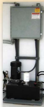
Hydraulic Pump System with control panel
