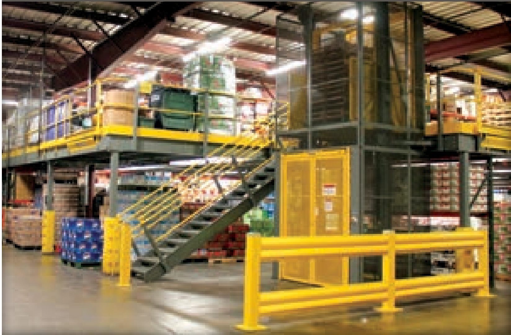
Baker Distributing is using the full complement of Wildeck® products to raise safety and increase production. The new mezzanine platforms, vertical reciprocating conveyors (VRCs), safety gates and guard rail at its two Vermont facilities are allowing Baker Distributing to better adapt to changing industry trends.
